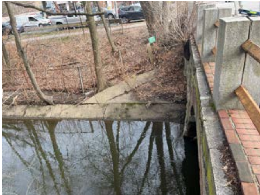
Photo 14. CSO outfall CAM-002 downstream of Massachusetts Avenue.
