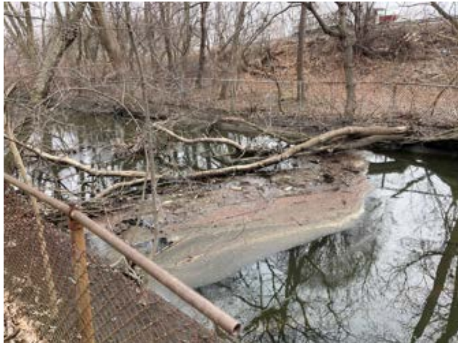
Photo 10. Typical debris jam in Stream Segment 2.
