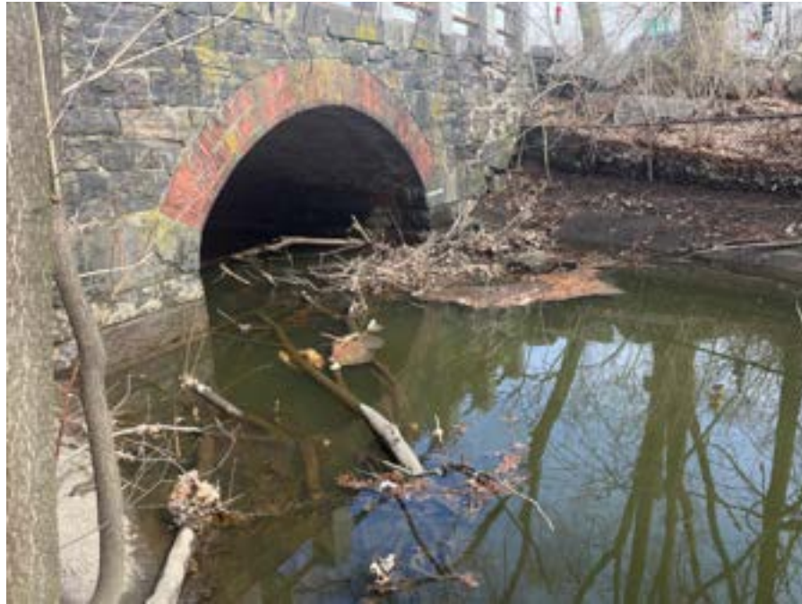
Photo 11. Massachusetts Avenue inlet of crossing structure, with debris jam.
