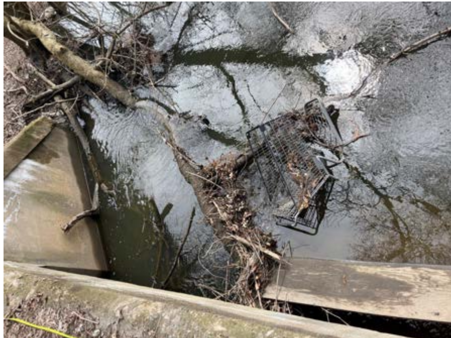
Photo 8. Concord Turnpike debris jam at inlet of crossing structure.
