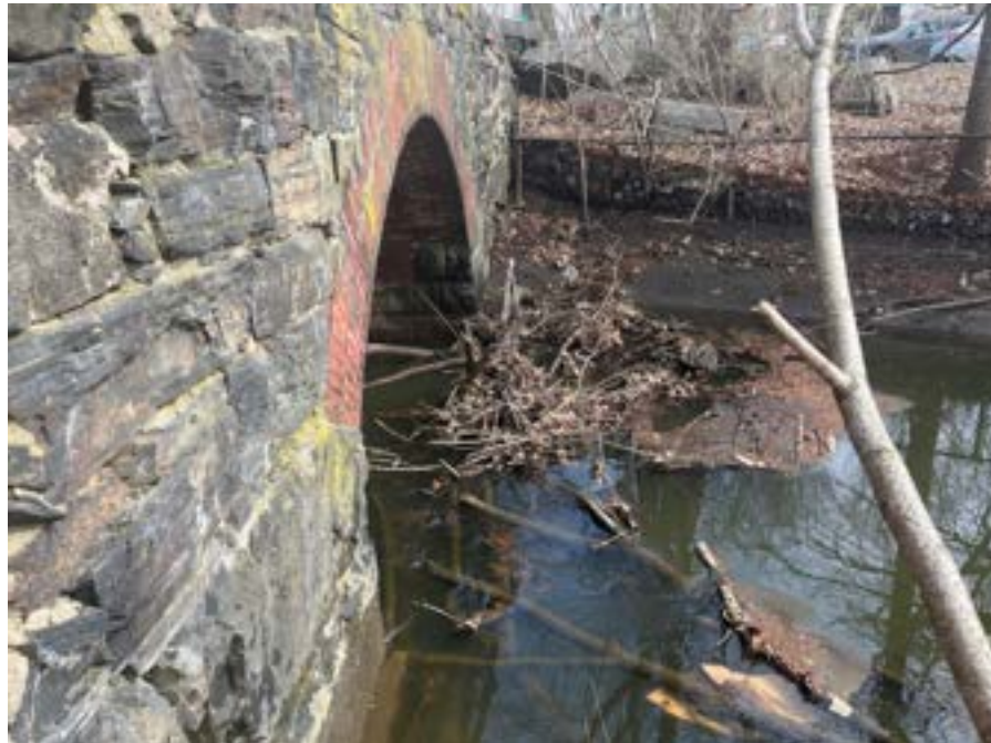
Photo 12. Debris jam at Massachusetts Avenue inlet.
