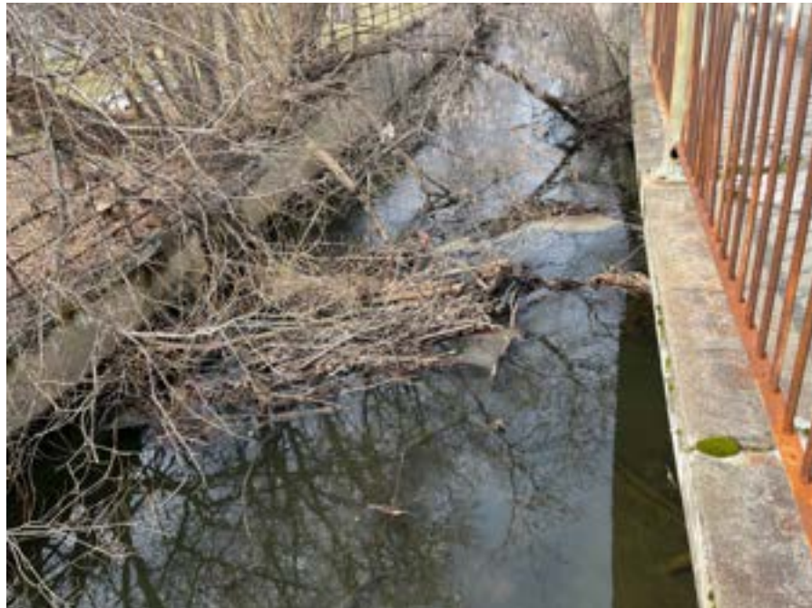
Photo 22. Typical debris jam in Stream Segment 4.
