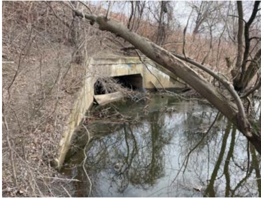
Photo 7. Concord Turnpike inlet at crossing structure, with debris jam
