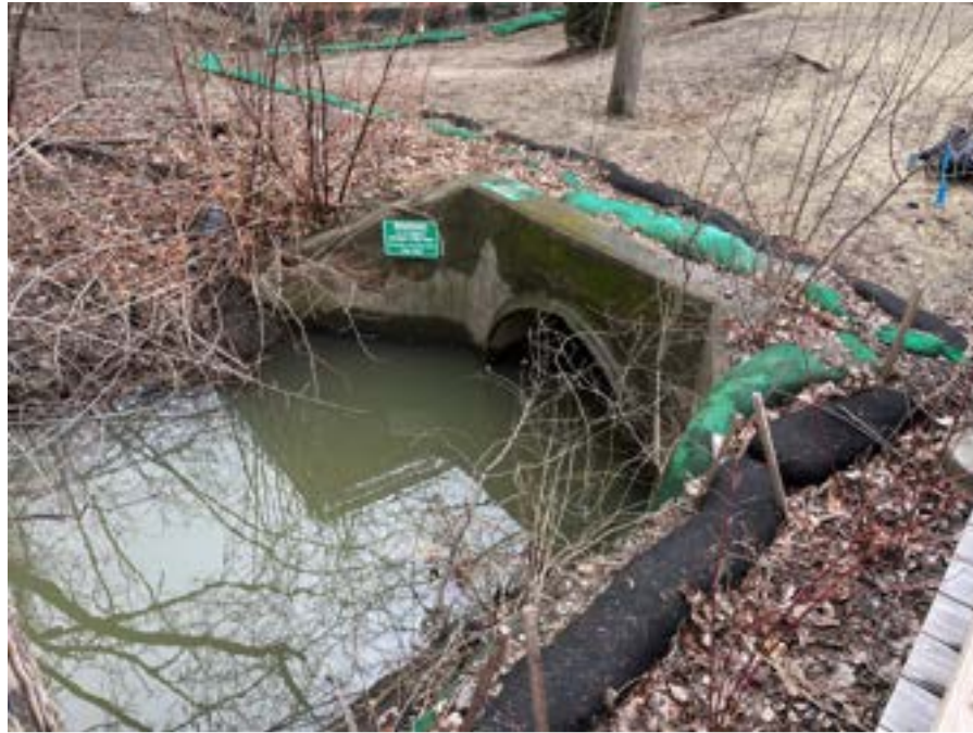
Photo 1. CSO Outfall CAM-401A at upstream extent of study area.
