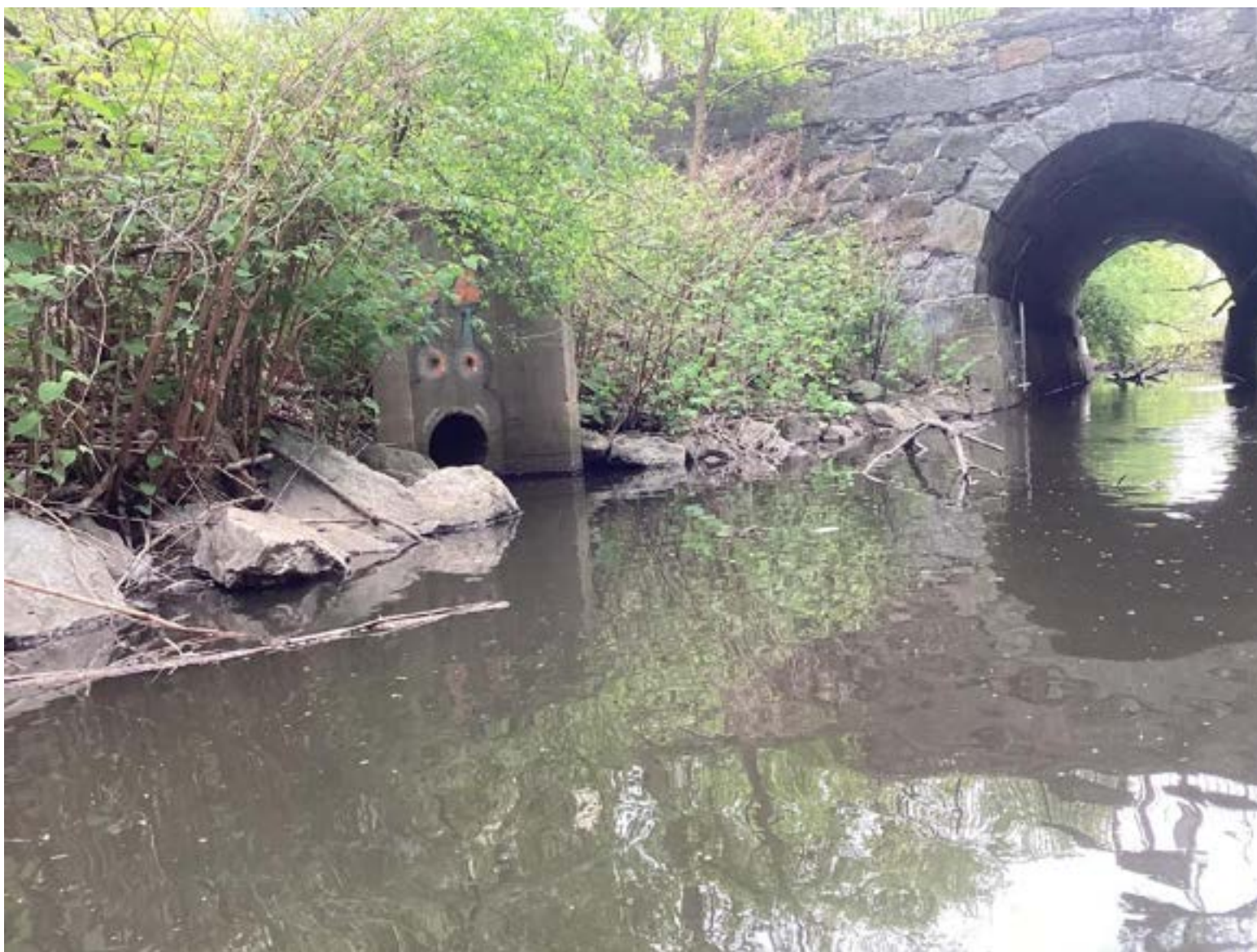
Figure 16. Reach D. Looking upstream towards the bridge at Broadway and river right bank. The stormwater drain on the river right bank is surrounded by concrete rip rap and the invasive Japanese knotweed.
