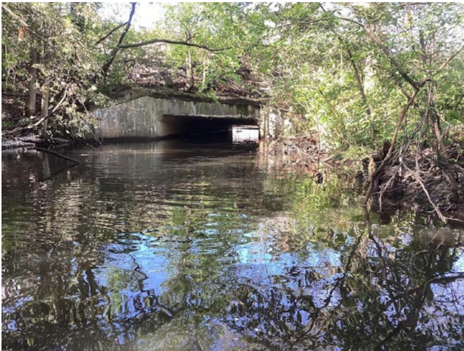
Figure 1. Reach A. Looking upstream at the Rt 2 Bridge with trees and shrubs growing on the concrete banks.
