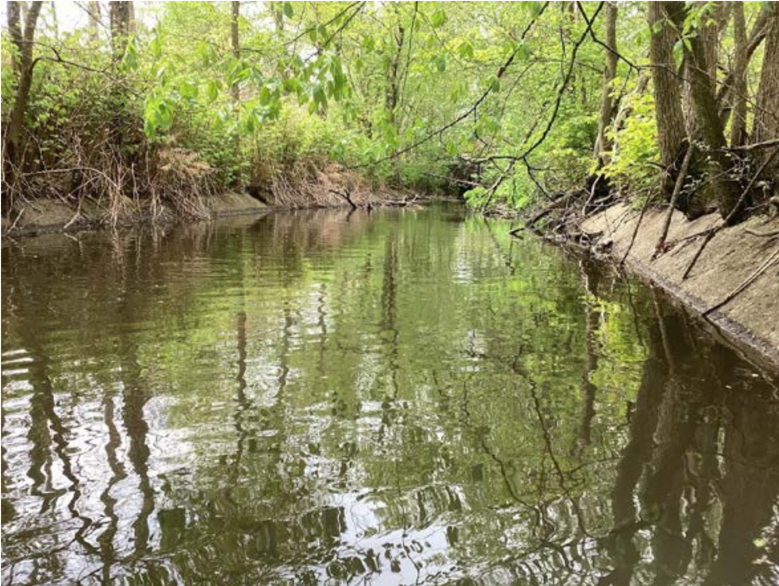
Figure 6. Reach B. Looking downstream. Note the invasive Japanese knotweed growing on top of both concrete banks.
