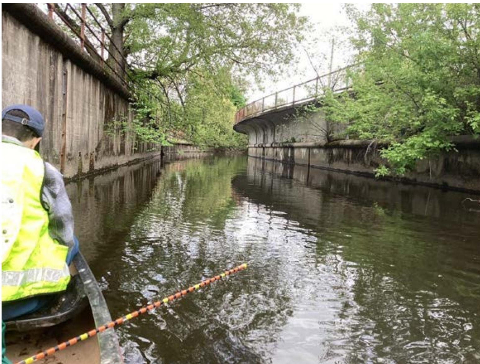
Figure 13. Reach C. Looking downstream at the vertical concrete wall on the left below St. Paul's Cemetery and the vertical and overhanging concrete walls on river right. Note the trees growing out of cracks within the concrete walls on river right.
