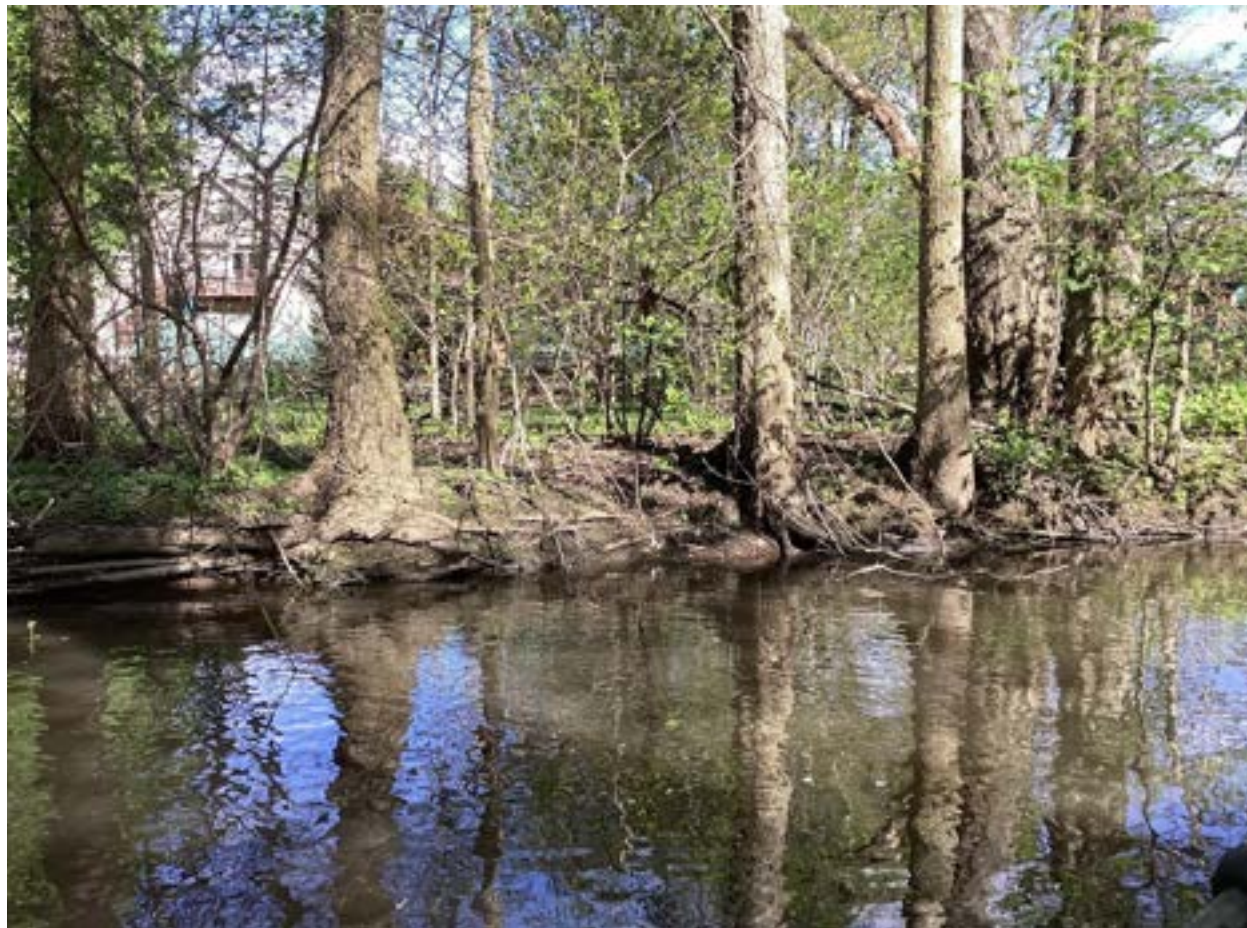
Figure 6. Riparian vegetation overtopping concrete banks on river left in Reach A.
