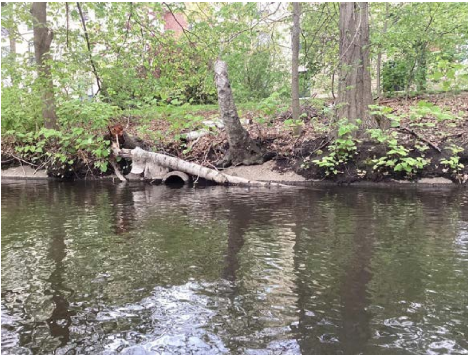
Figure 9. Reach B. River right bank with stormwater drain. Throughout this reach, tree roots and topsoil overtop the concrete banks.
