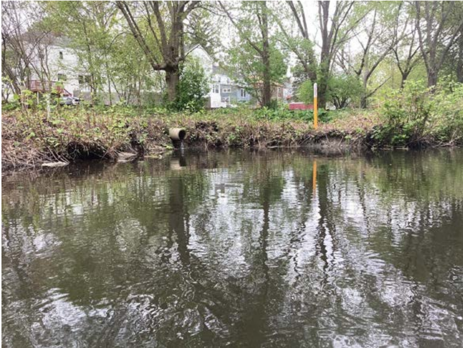
Figure 18. Reach D. Looking downstream towards river left at a stormwater drain and bank erosion.
